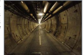
The service tunnel
