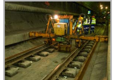
The new rails are positioned next to those to be replaced. A machine removes the old rails and puts the new ones in place in one operation.
