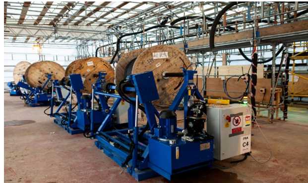
Figure 17: External jointing facility
