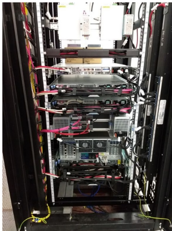
Figure 7: IT hardware and systems
