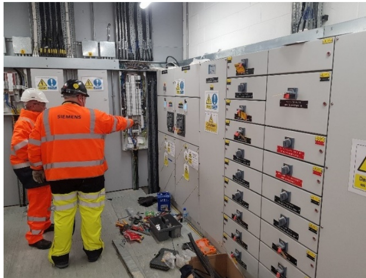
Figure 6: Low voltage distribution panels
