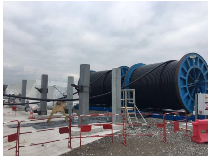
Figure 8: HVDC cable drums
