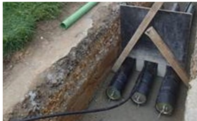
Figure 20: Underground AC cables in the UK
