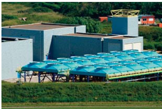
Cooling plant in Sangatte (FR)
